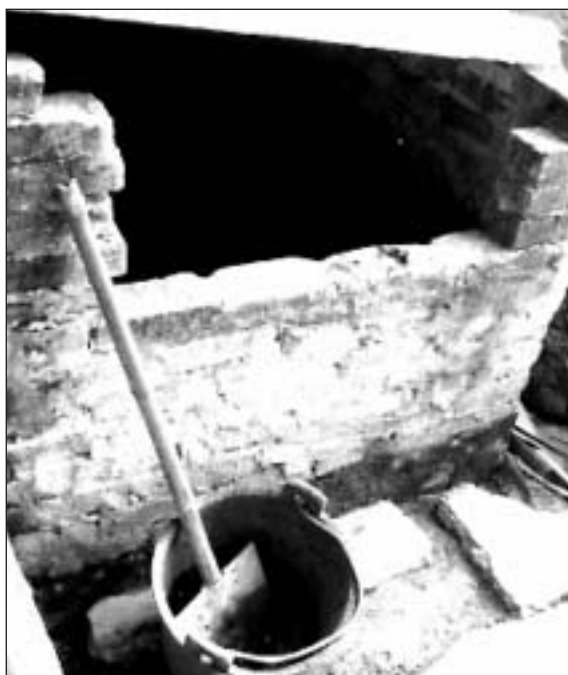
Figure 7: Scraped slurry pit, farm type III
