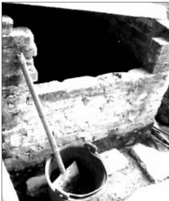
Figure 7: Scraped slurry pit, farm type III
